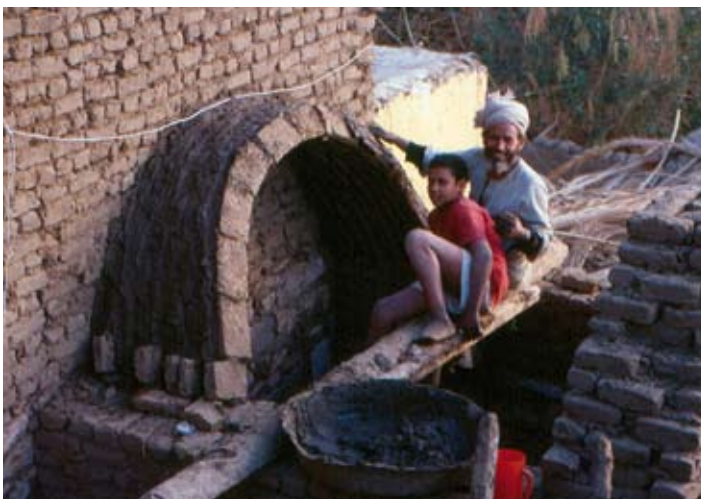
Oral transmission of practitioners' knowledge: construction, without centering, of a Nubian barrel vault using sun-dried bricks, Elephantine, Egypt, 2001 (photo by D. Kurapkat)
